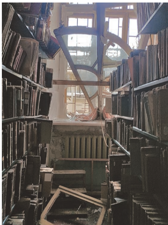
FIG. 4. The Karazinsky Library, which was damaged by the war. Photo by Iryna Zhuravlyova
